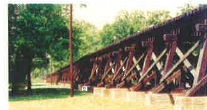
Figure 37: This rail trestle in Harpers Ferry NHP is an example of how rail structures can be integrated into the park setting as both interpretive and aesthetically pleasing features. (WRT)
