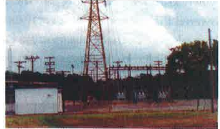
Figure 30: The existing structures of the substation could be partially screened by trees, shrubs, and walls. (WRT)
