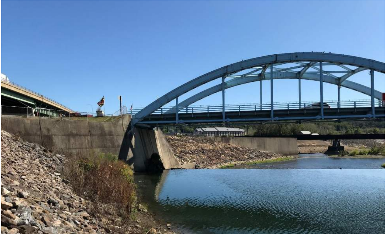
Existing floodwall and dam on river left (Maryland). Proposed location of trail underpass adjacent to water feature drop.
