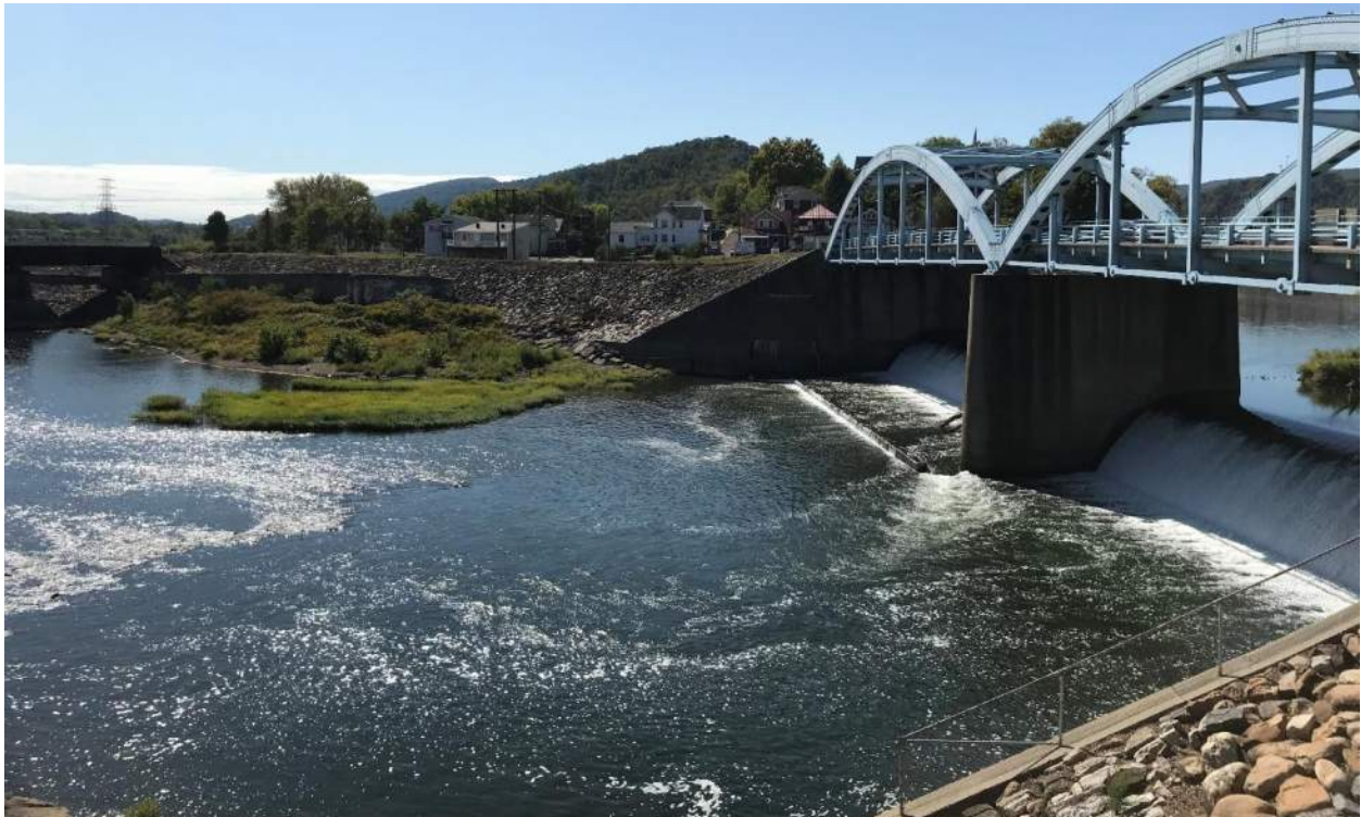
View of Ridgeley Flood control wall and Bridge Street Crossing. Proposed trail intersection with Bridge Street.
