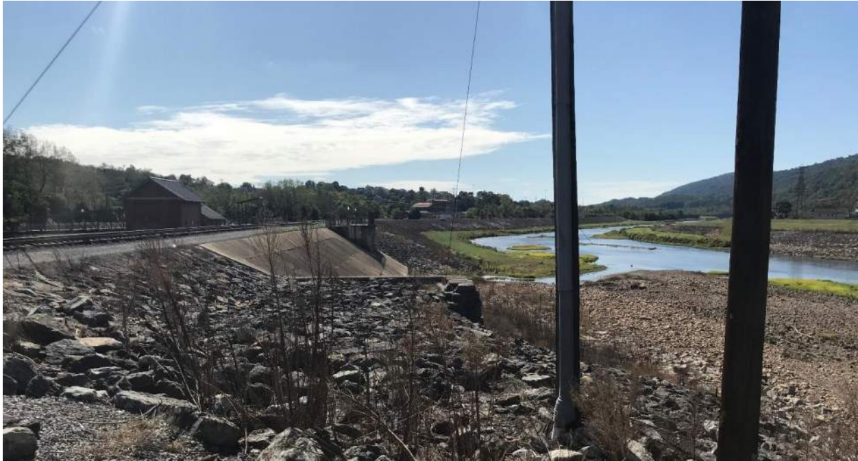
Existing flood wall River Left (Maryland side) downstream of railroad trestle. Proposed area for overlook and stair access to river trails.
